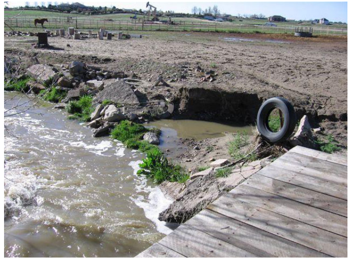
Erosion around private pasture-access bridge in Adams County following large July 2004 storm event.
