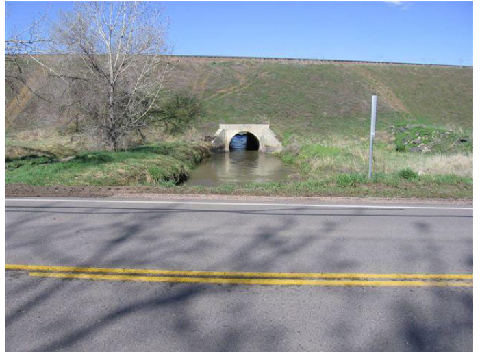
Undersized culvert at the Union Pacific Railroad embankment near Colorado Blvd. provides inadvertent detention of flows in Big Dry Creek.
